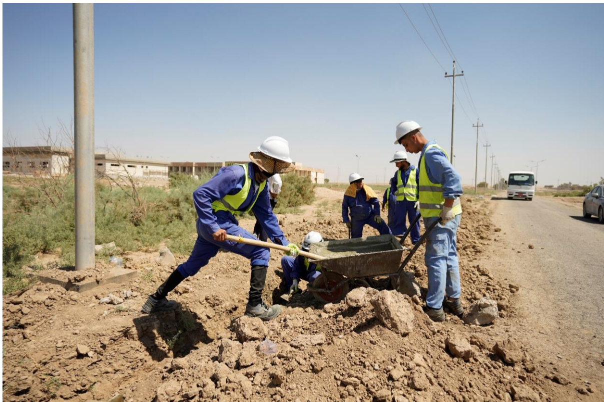
Construction workers installing drinking water pipeline through the project's interventions at Nineveh Governorate, by Zanyar Qadir, © ILO, 2022
